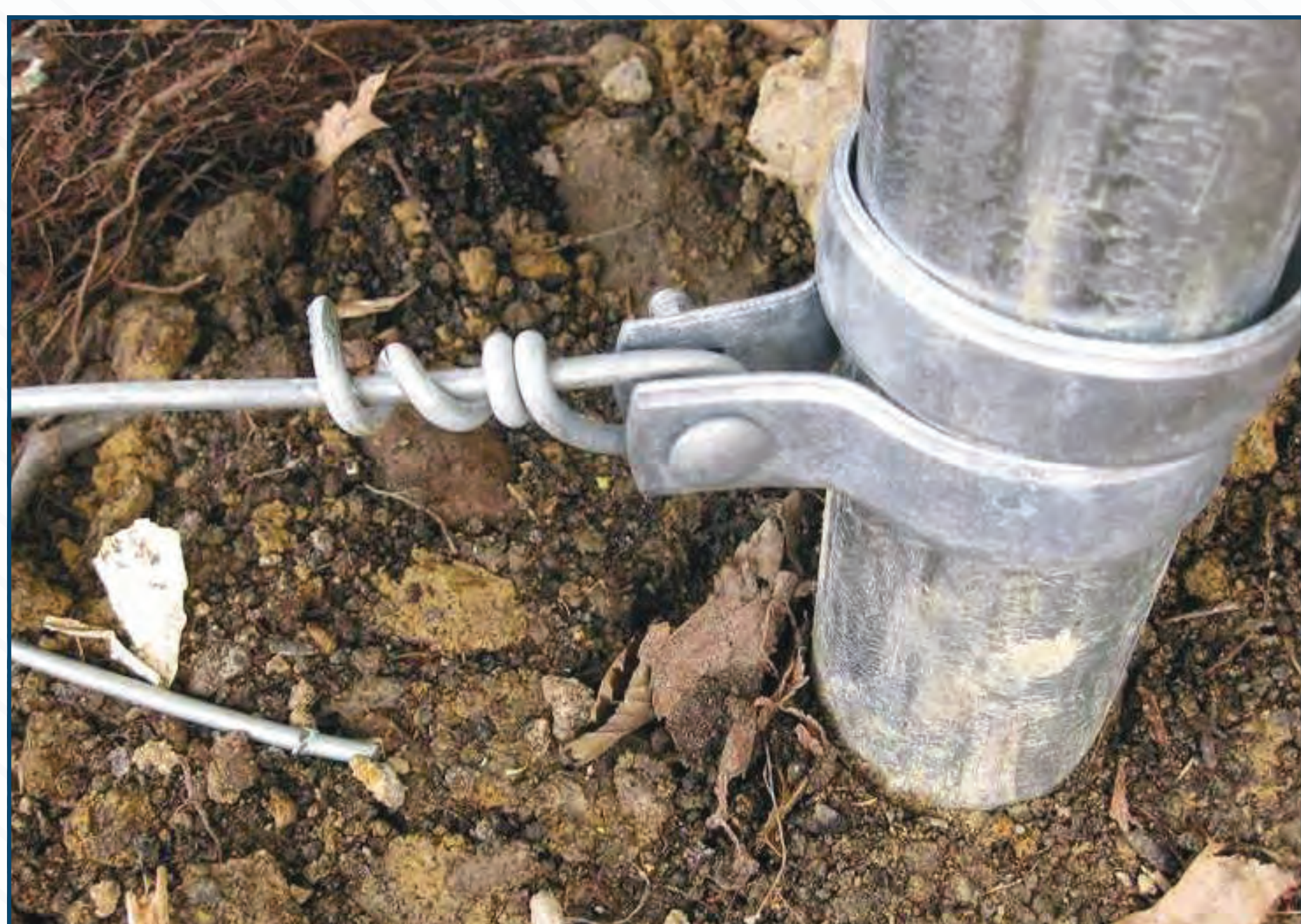
Tension band reinforces chain link fence
